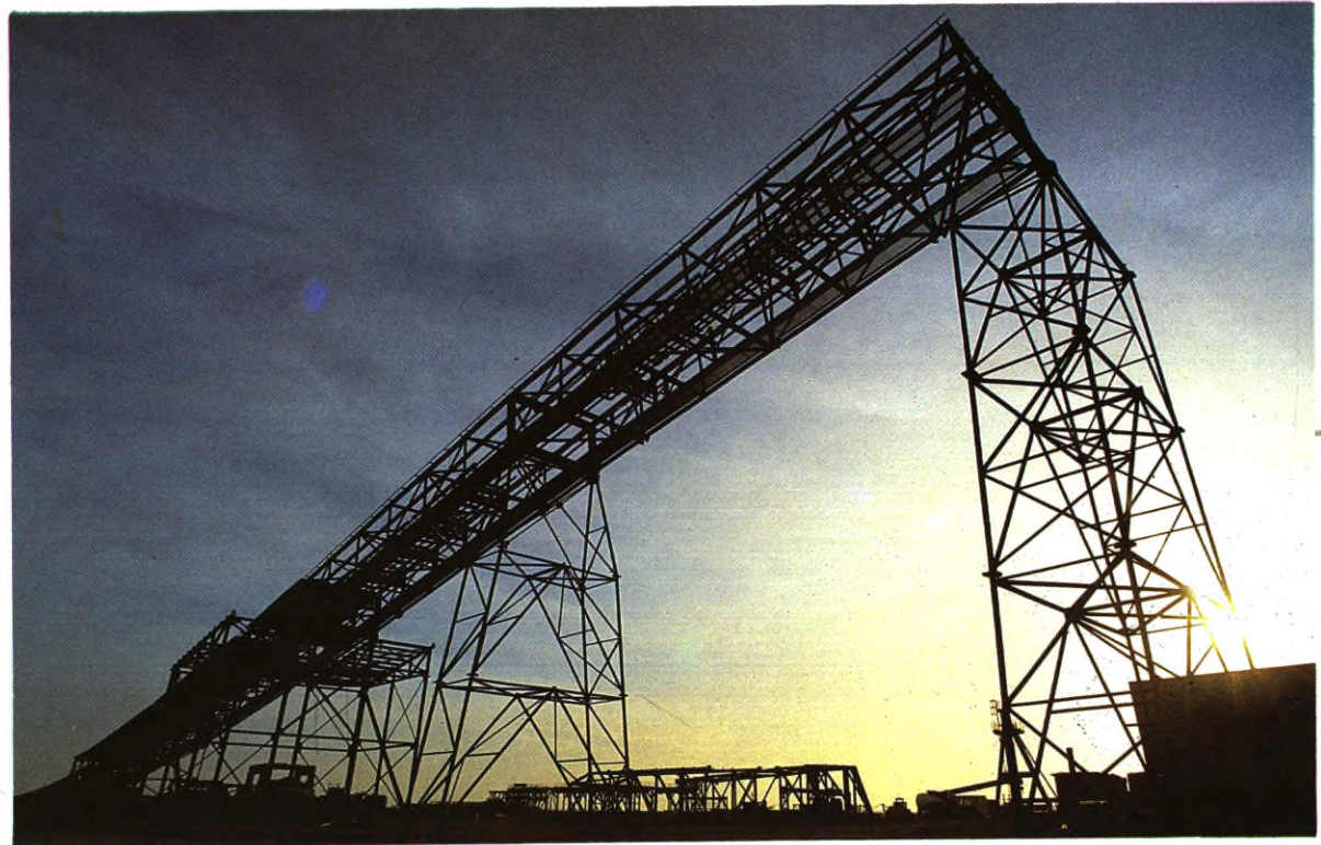
Structure of the coal transporting band in the port.
