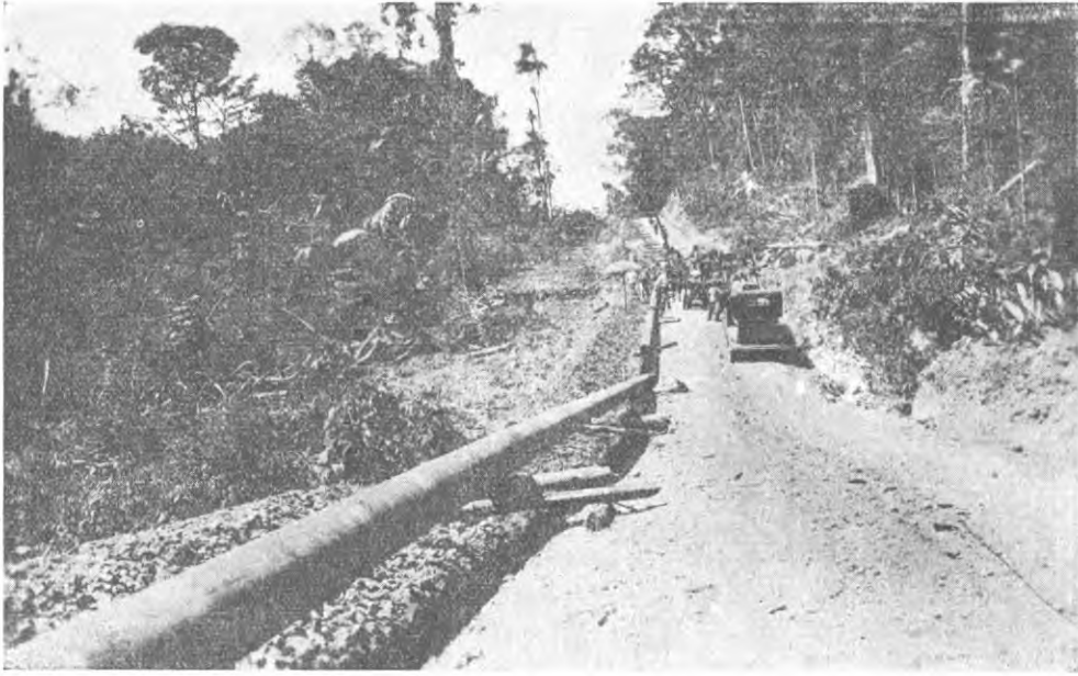
Fig. No. 48.—The Pipe-line of the South American Gulf Oil Company is being constructed.
