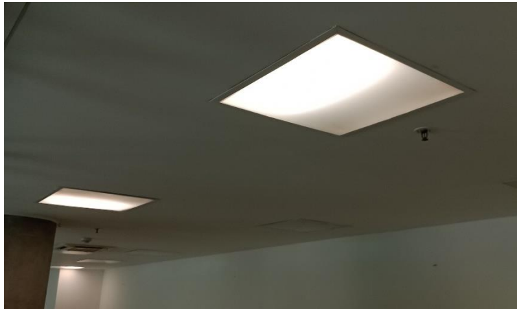
Panel LED 60x60 con fallas Ilustración 83 Panel LED 60X60
